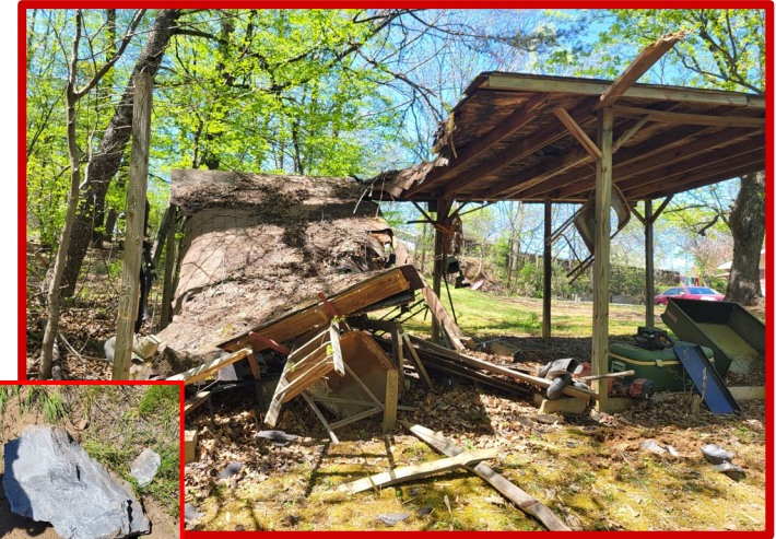
Flyrock damaged shed - April 2023
